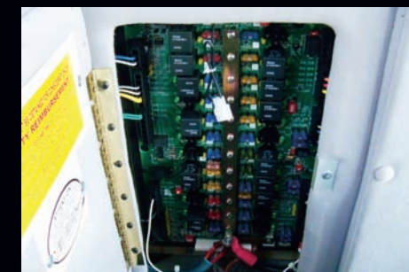
Printed electrical circuit board with LED trouble-shooting lights
